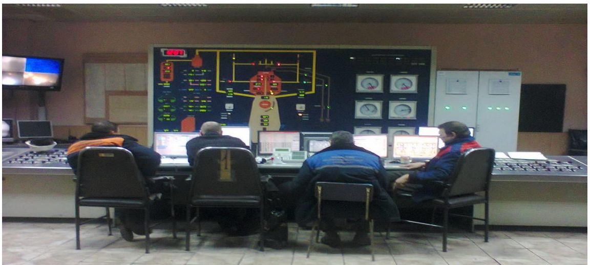
Fig.4. Central Control Console before reconstruction
